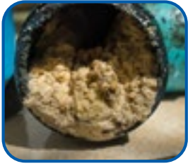
Look at all of that grease!
